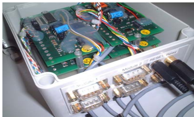
Battery Management System
